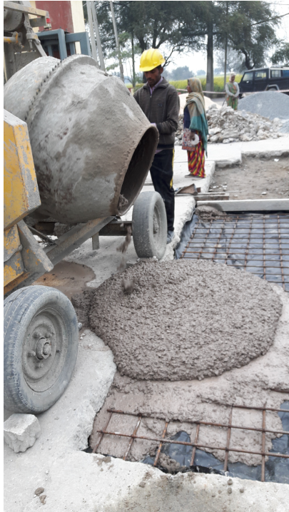
Road being built at the truck exit gate of JK Lakshmi cement plant
