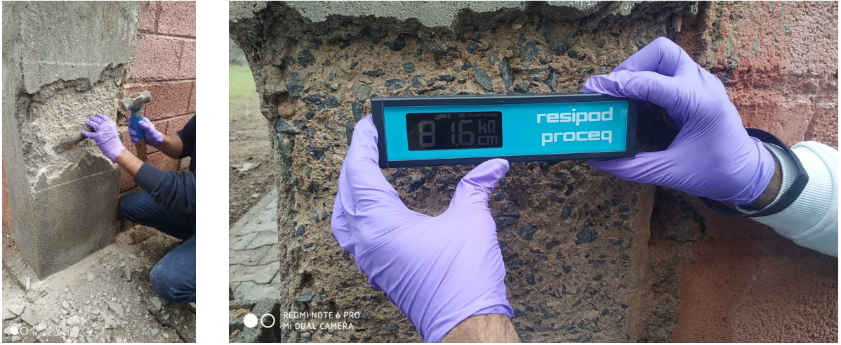
Figure: 6 left) breaking of the plaster from over the concrete and right) resistivity measurement on the exposed column surface.
