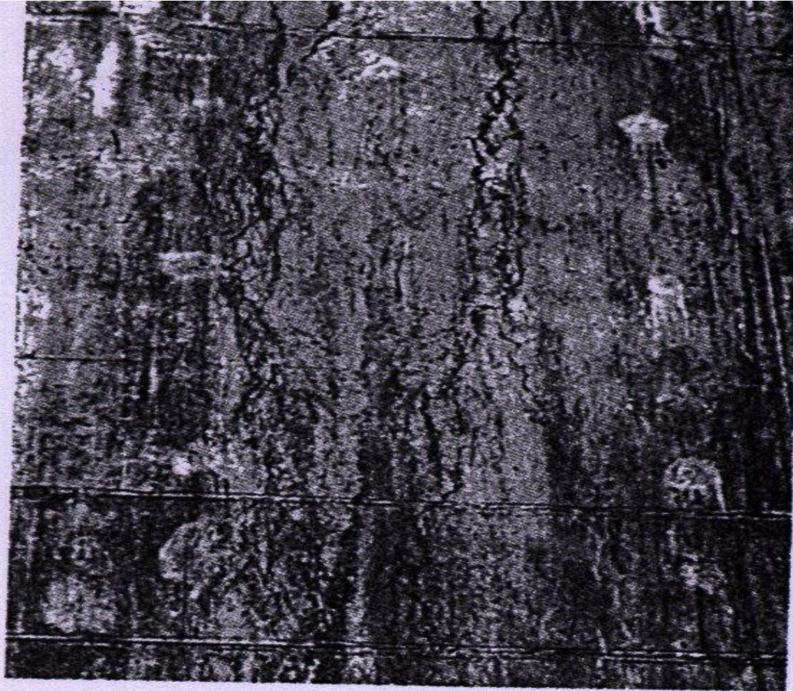
Fig. 7.6.3—Sand streaking caused by heavy bleeding along form
