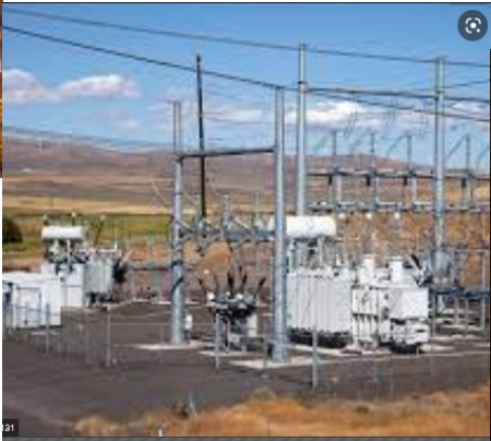
Delhi-Faridabad Electric Sub-station 1885
