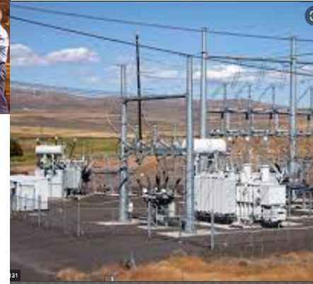
Delhi-Faridabad Electric Sub-station 1885
