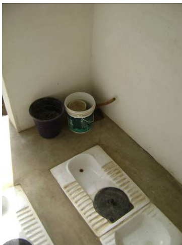
Figure15. Squatting type urine diverting dry toilet with two chambers (Photo: Dr. Lucas Dengel)
