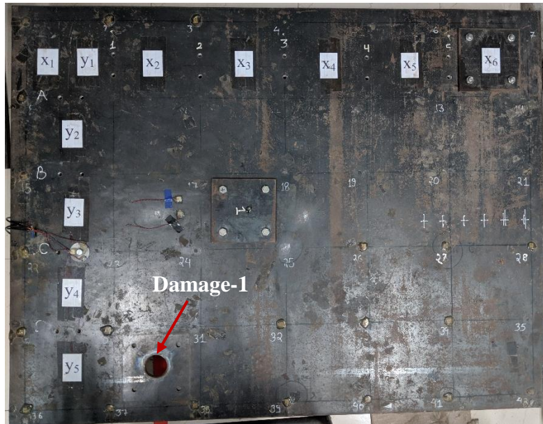
Figure 4.5: Steel plate with damage location 1
