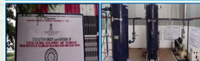
100 Nm 3 /day cow dung based compressed biogas (CBG) plant at Sharda Vihar, Bhopal, Madhya Pradesh
