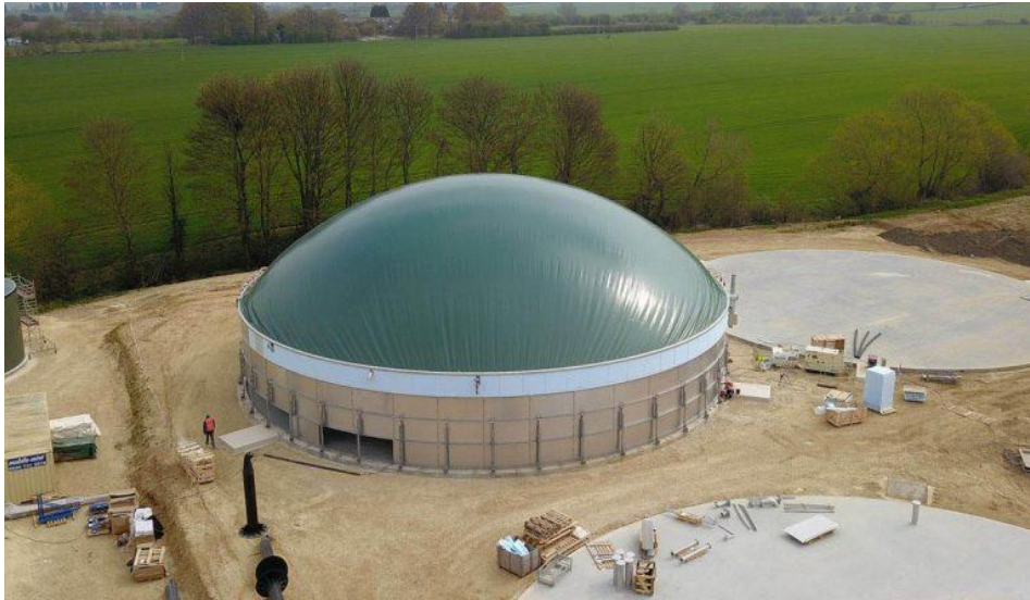
Fig. Weltec Biopower Plant (Source: Weltec Biopower)
