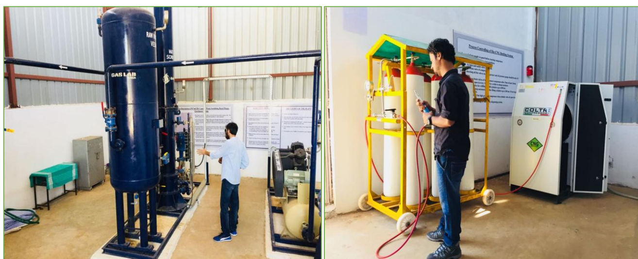
Fig. 1. Water scrubbing technology installed for CBG production at Sharda Vihar Jankalyan Samiti, Bhopal, Madhya Pradesh.
