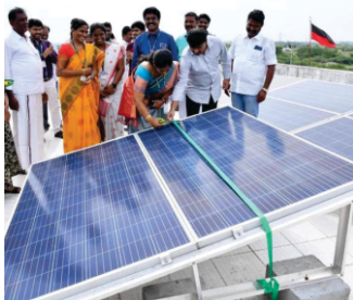
SOLAR ELECTRIFICATION STATION
